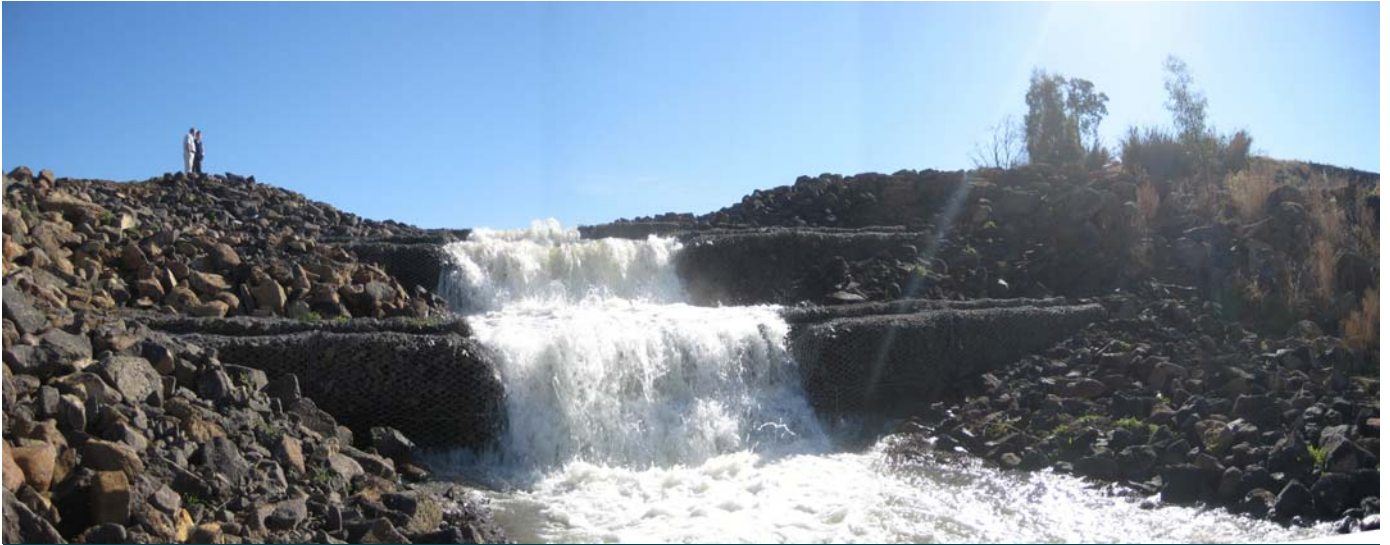
Fully Functional Gabion Drop Structures
