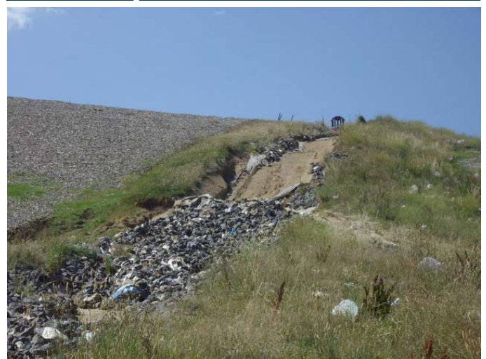
Loose Rock Washed Down The Channel
