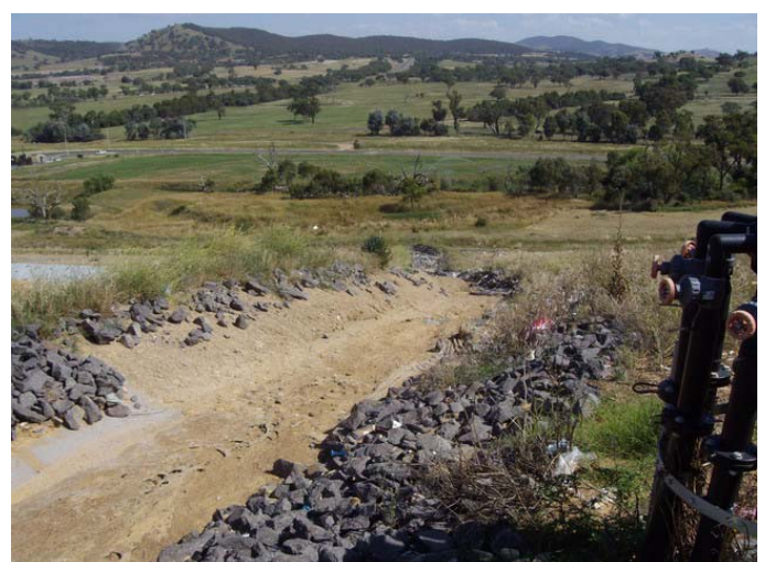
Close Up Of The Damaged Loose Rock
