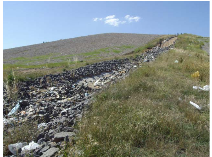
The Storm Damage To The Loose Rock
