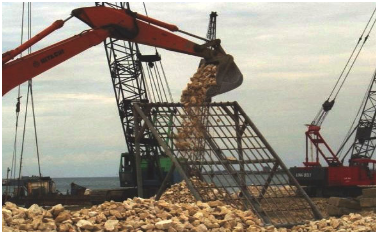
Figure 3. Stringent control using sieving to ensure secondary armour rock gradation meets the requirements.
