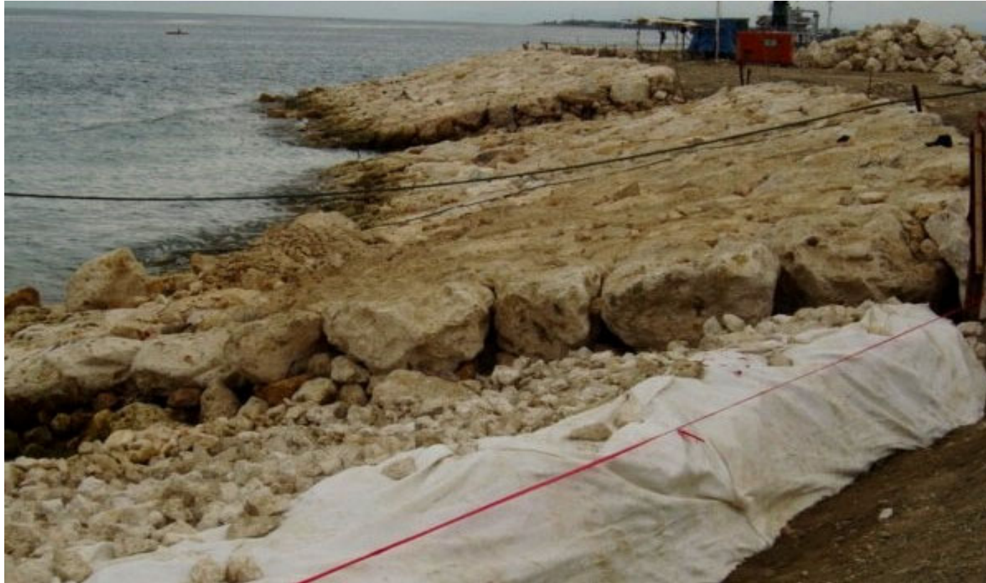
Figure 5. Overview of high strength woven geotextile filter with armour rock protection system.
